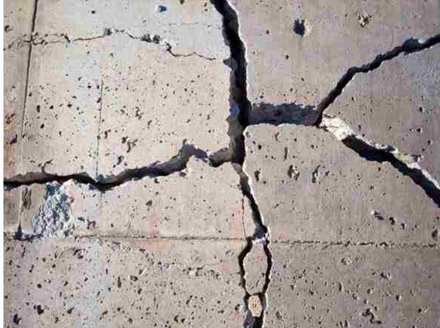
Figure 1.1 – Discontinuous deformation field in a reinforced concrete beam (courtesy of http://www.anatech.com/capabilities/material-behavior-modeling/reinforced-and-prestressed-concrete/ )
